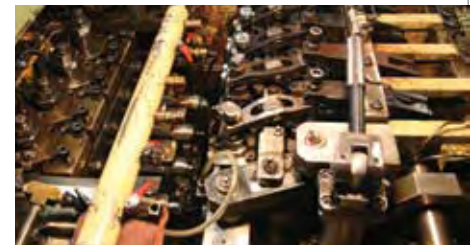
Inside a 4-die header. The punches, visible at center, move horizontally, left to right. The four slotted bars to the right of the punches are part of the transfer mechanism. The dies lie below.
